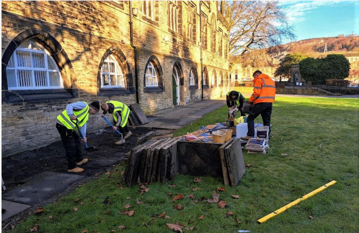
Apprentice Builders, Decorators and Joiners from Calderdale College spent a day at the Minster.
