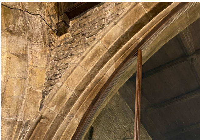
Water ingress damage in chapels
